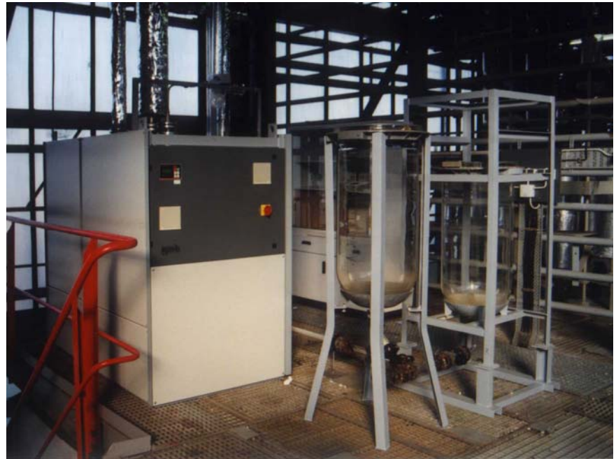
↑ platform 1: heating steam generator
